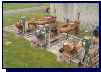
Equalization Basin Pump Station
