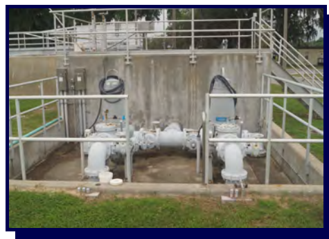
RAS/WAS Pumping System
