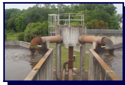
Kruger Oxidation Ditch Flow Splitting Structure
