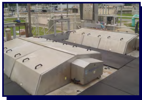
Tertiary Filtration System
