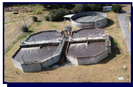
Kruger Oxidation Ditches
