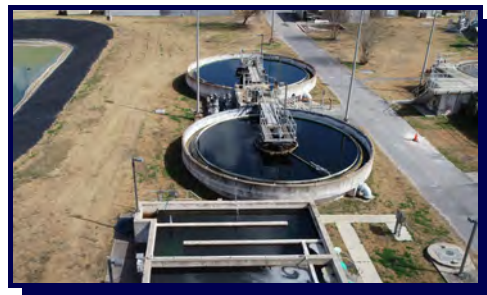
Secondary Clarifiers (40-foot diameter)
