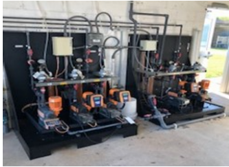
Chemical Pump Pic
