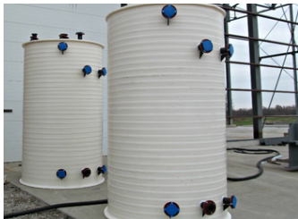
CL2 Tank Pic
