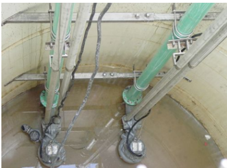
Riser Pipe Pic
