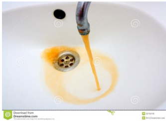
Iron filter Pic
