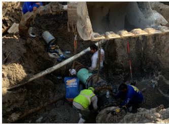
Pic of 16" Main Break
