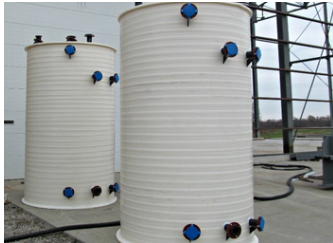
CL2 Tank Pic
