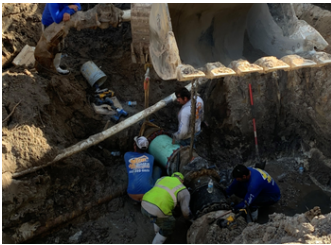
Pic of 16" Main Break
