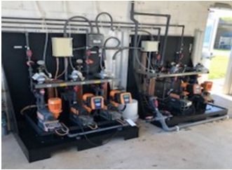
Chemical Pump Pic
