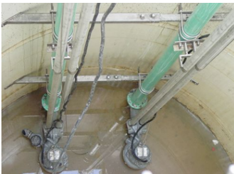
Riser Pipe Pic
