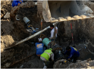
Pic of 16" Main Break
