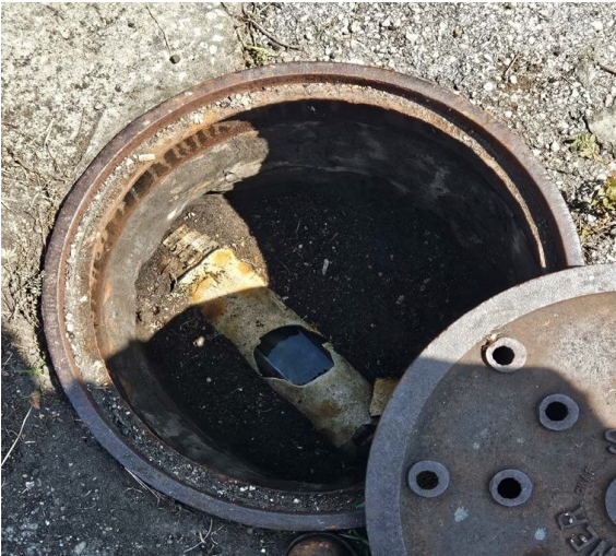
INFILTRATION FOUND SMOKE TESTING
