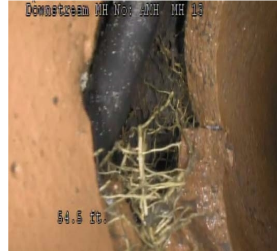
DAMAGED GRAVITY MAIN FOUND DURING ROUTINE INSPECTION
