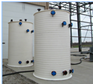
Chemical Tank Pic
