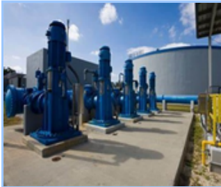
R-12 Pump Station
