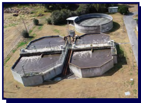
Kruger Oxidation Ditches
