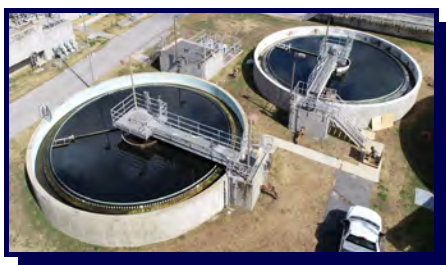
Secondary Clarifiers (50-foot diameter)
