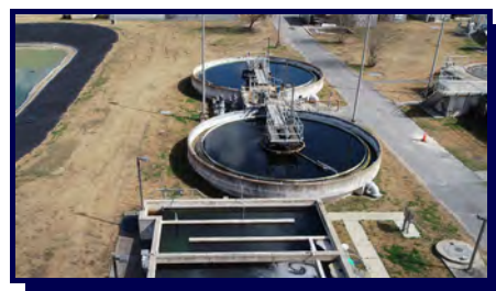
Secondary Clarifiers (40-foot diameter)
